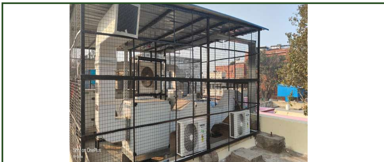
Figure 6.16: Example of fully controlled Mechanical Ventilation – AHU/ HVAC system in JLNMH, Agra.
