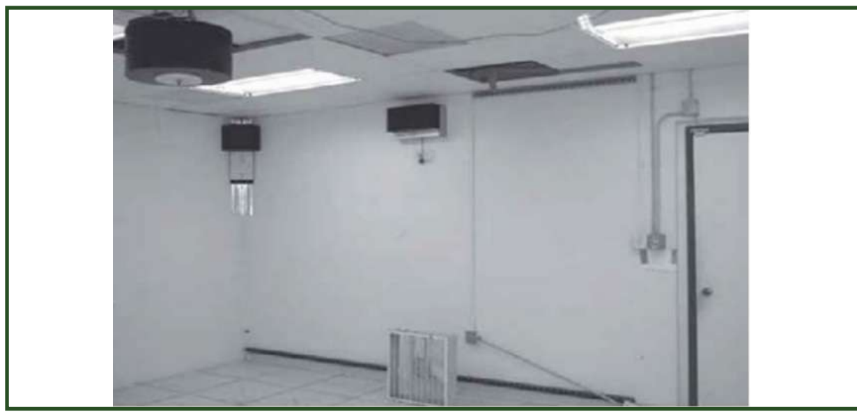
Figure 6.32C: Different types of ceiling, corner and upper room GUV fixtures
