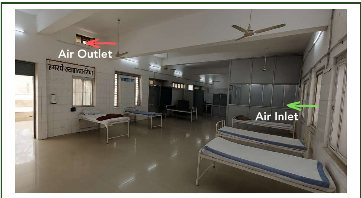
Figure 6.12: Example of mixed-ventilation at DR-TB ward in Chhatarpur, Madhya Pradesh
